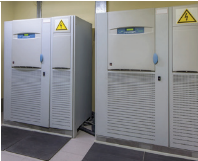
UNINTERRUPTIBLE POWER SUPPLY SYSTEMS
