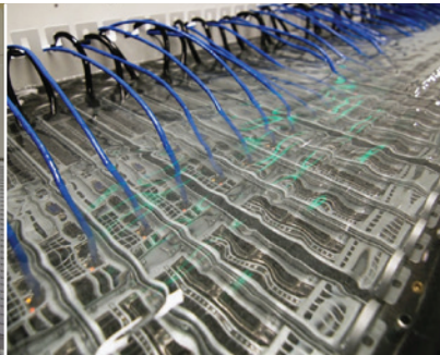
LIQUID COOLING SYSTEMS
